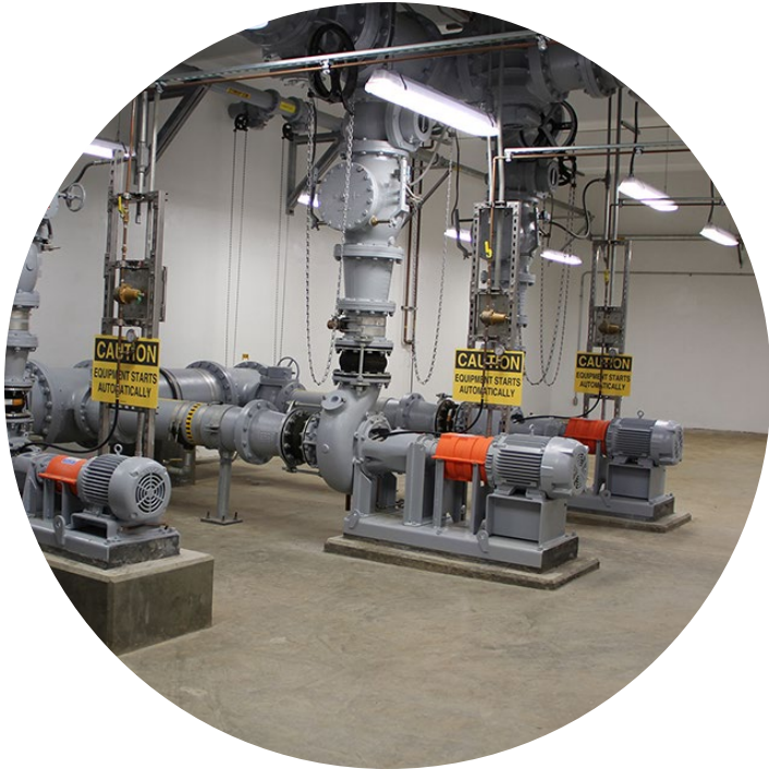
New Return Sludge Pump Station serving the new third treatment train with space for a future fourth train.
