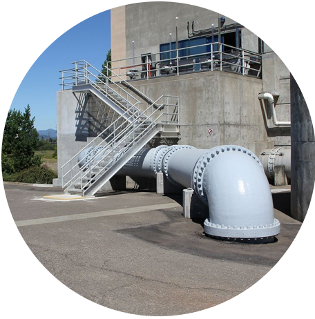
42-inch diameter ductile iron pipe added to the existing Headworks to split flow to the new aeration basin.
