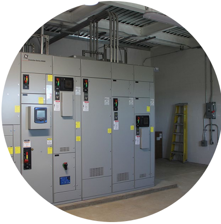
New motor control center and energy efficient variable frequency drives serving the new treatment process.
