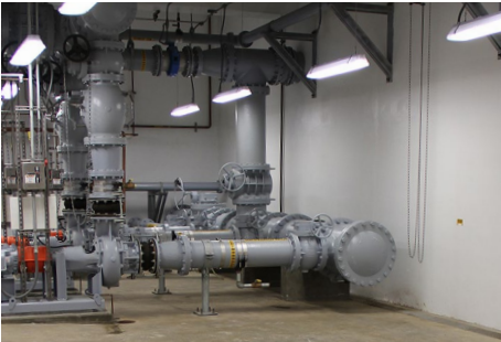
Return Sludge Pumping Station
