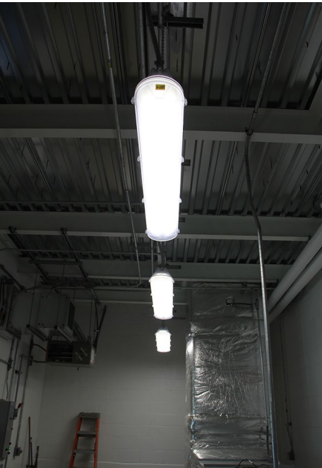
LED fixtures used for all interior and exterior lighting.
