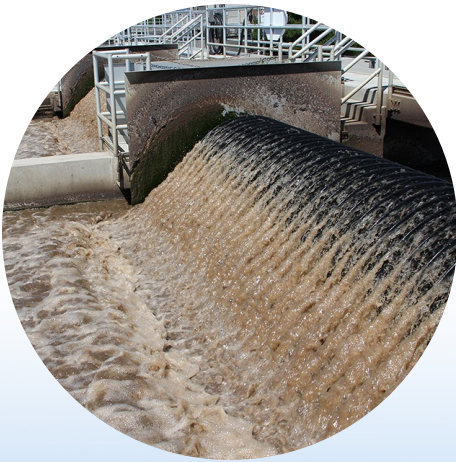
Optimized aeration basin matching the size of the existing basins but with an additional 10-percent treatment capacity.
